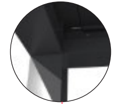
NO VISIBLE SCREWS CONNECTING THE GUTTER WITH THE BASE OF THE PERGOLA
